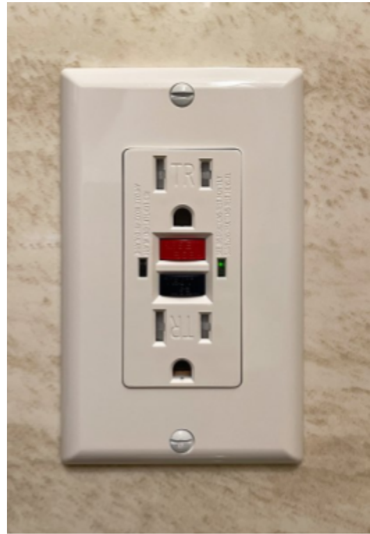
Figure 1: A typical North American residential GFCI outlet, installed (Kurtovic, 2021)
